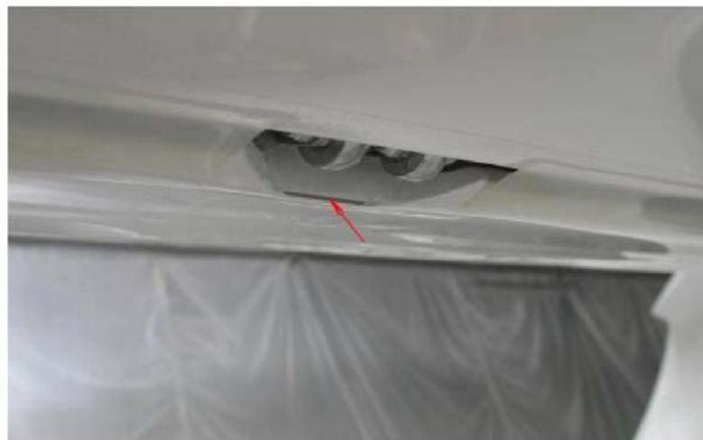
Fig. A: Inspection area: Trim tab control horn attachment point (Seen from underneath the stabilator)
